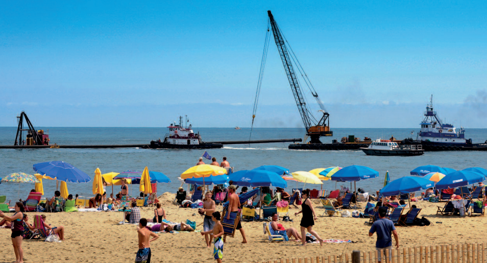
Beach replenishment work takes place in Rehoboth in 2012. Supporters say pumping sand to widen beaches and fortify dunes helps offset erosion and lessens damage during storms.
